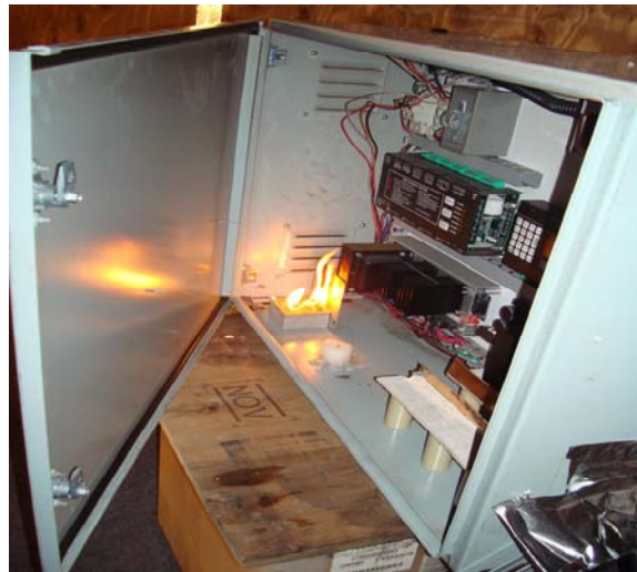
Figure 9 – Vented enclosure with copper bus bars
